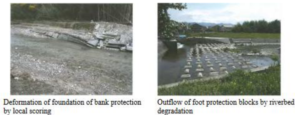
Figure 17. Deformation of river structures due to riverbed degradation/local
