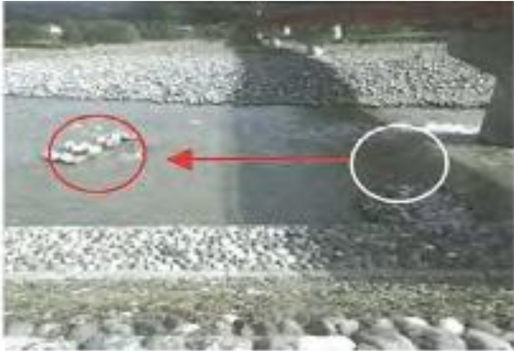
Figure 21. Outflow of concrete block of spur dike
