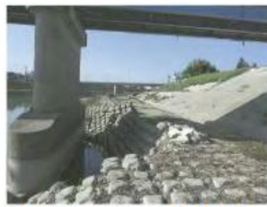
River bank erosion near a bridge pier
