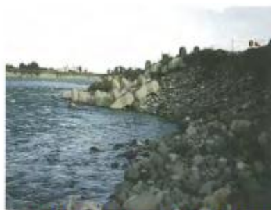
River bank erosion at the curved reach
